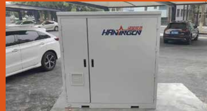
50kW/100kWh User-side Energy Storage for Power Training Center
