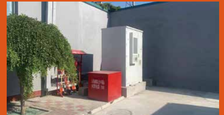
13MWh All-in-One Optical Storage and Charging Project
