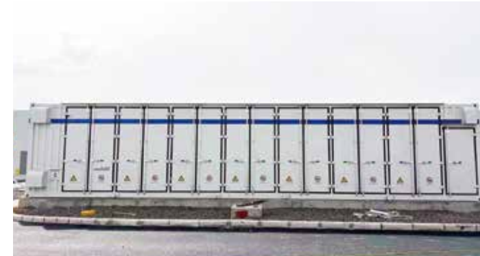
5MW/10MWh User-side Energy Storage for Haier Refrigerator Factory
