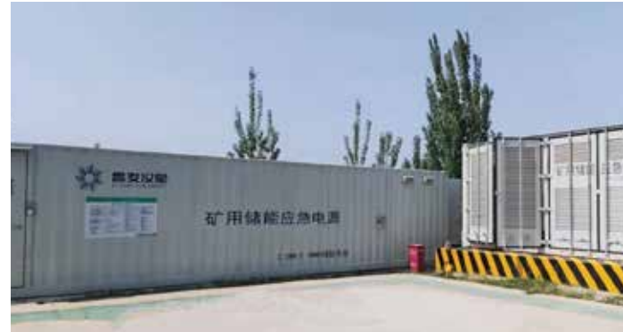
2.5MW/2.5MWh Energy Emergency Power Supply For Anju Coal Mine
