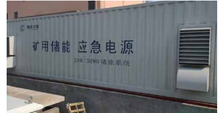
2MW/3MWh Energy Storage Emergency Power Supply for Hongqi Coal Mine
