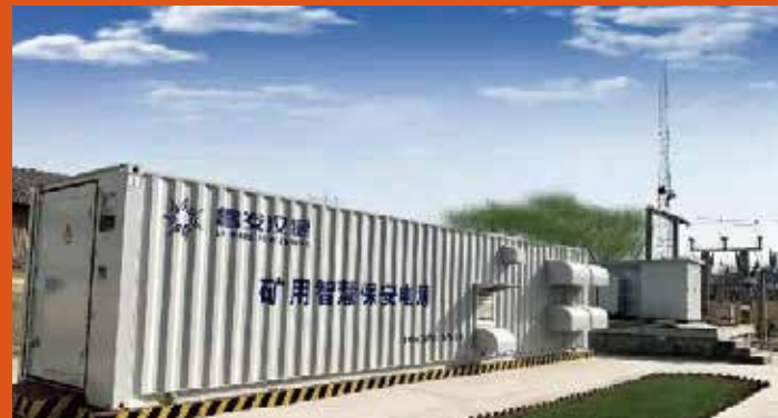
Henghe Coal Mine 2MW/4MWh Mining Smart Security Power Supply Project
