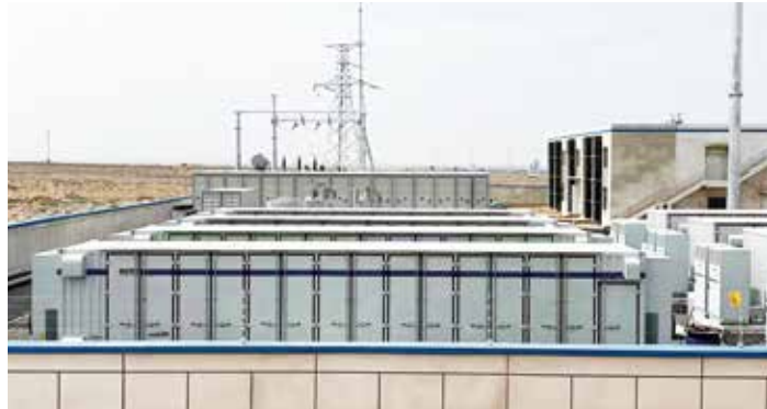
20MW/40MWh Energy Storage Power Plant
