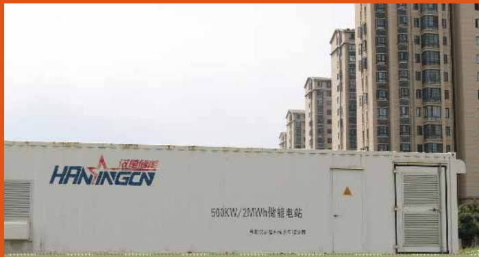
13MWh All-in-One Optical Storage and Charging Project
